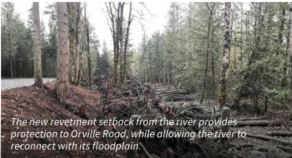
Another layer of racking logs and slash are applied to the anchored structures to cover the concrete dolosse and provide surface roughening to disrupt flow and slow velocity.
