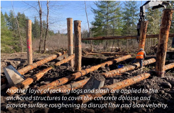
To build the engineered log jams, horizontal logs are manually anchored to the pile-driven vertical logs. The woody structures are stabilized by concrete dolosse that mimic large woody debris.
